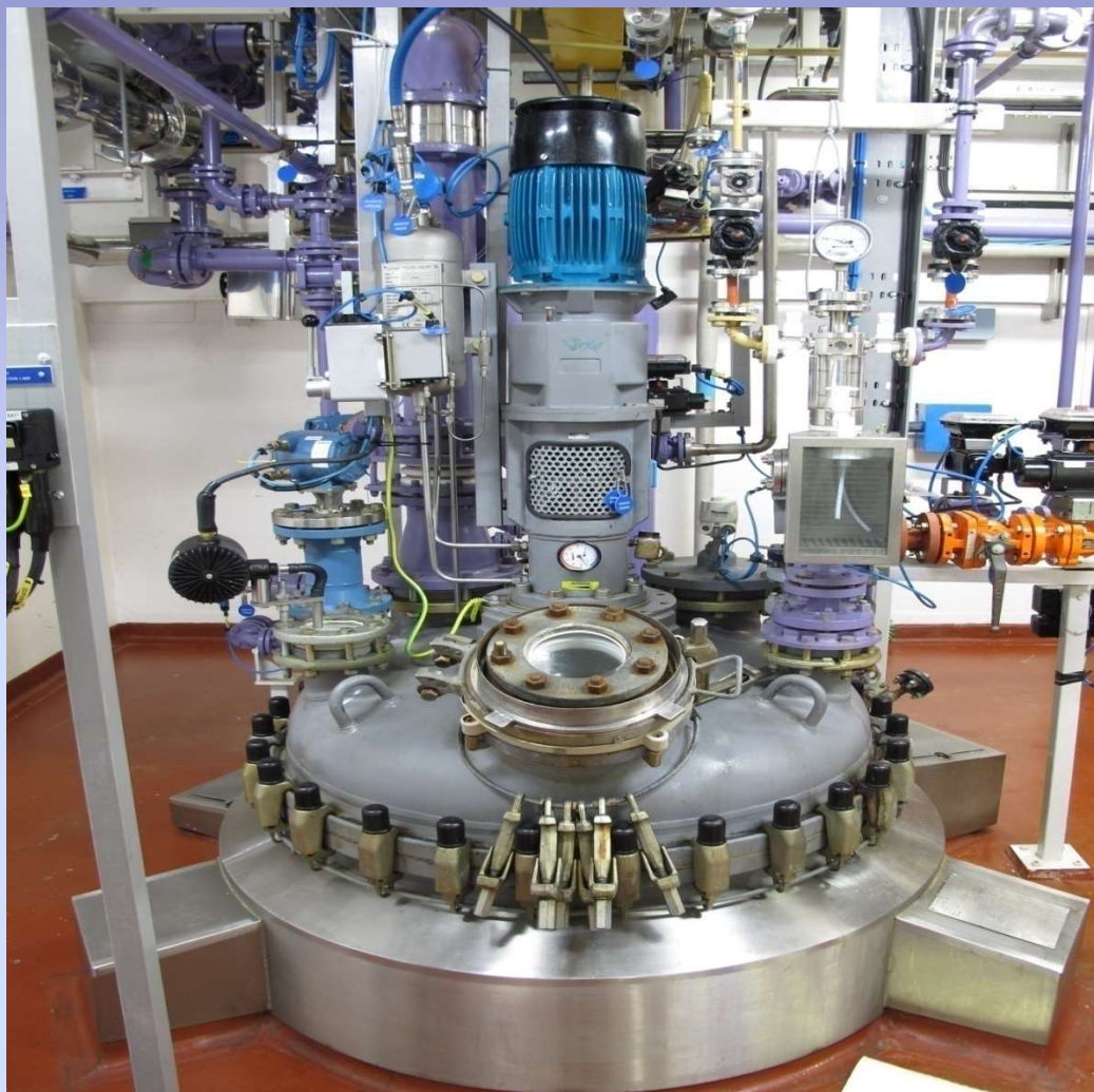
GLASS LINED REACTOR
